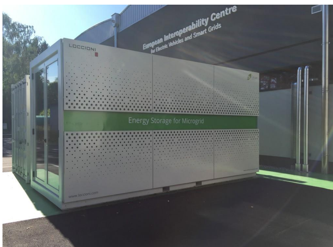
Fig. A – BESS at the SGILab of JRC in Ispra (VA) [130].
